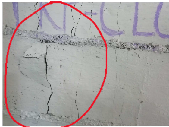
Fig.11. failure of mortar joint and micro cracks formation in fiber reinforced CLC prism
