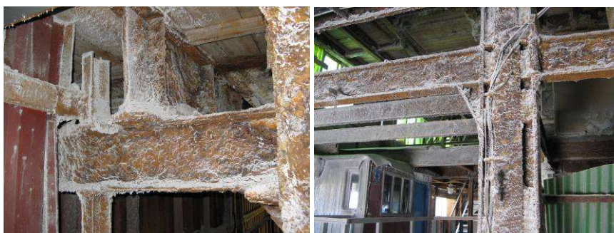
Fig. 3. View of the technical state of load-carrying beams and main beams of the frame
