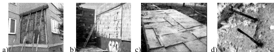
Fig. 12. Effects of the "hidden" construction defects in the joining of the layers: a), b) view of ZWS type walls after separation of texture layer [21, 26], c) view of inside surface of separated texture layer following the removal of mineral wool insulation [21], d) broken bars of hanger anchored within the texture layer [21]
