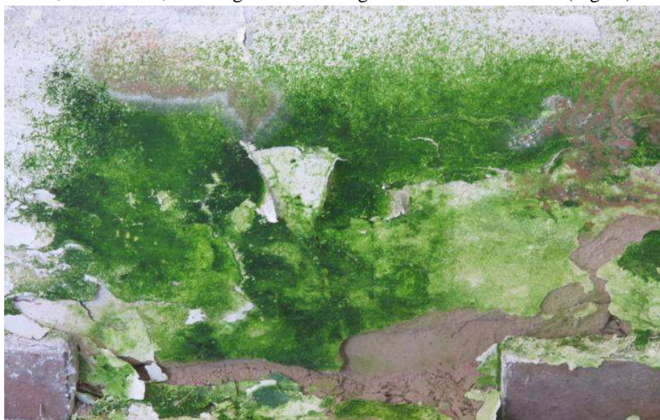
Fig. 1. Detail of the facade of the building with clearly visible biocorrosion
