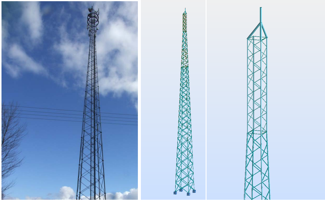
Fig.1. Photo (left), discretization of the entire structure (middle) and its top (right) in the FEM system ROBOT.
