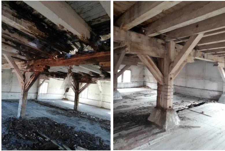
Fig. 5. Structural elements damaged by fire, uncontaminated section of building structure author archive
