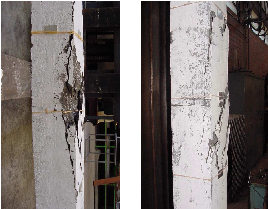
Fig. 11. Example of reinforced concrete pillars from geopolymeric concrete after the performed durability tests [28]
