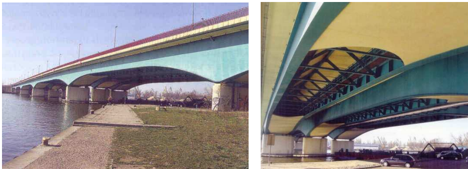
Fig. 12. Girder bridge of double composition over the Regalica river in Szczecin (Poland)
