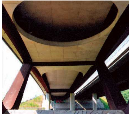
Fig. 11. View from below the RC slab in girder bridge of double composition over the Oder river in Stary Bohumin (The Czech Republic)
