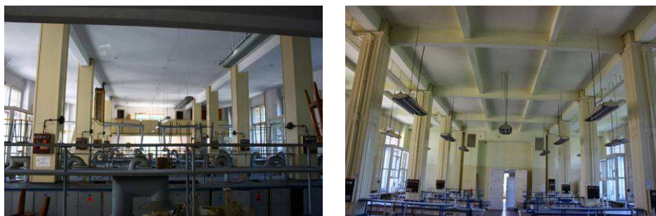
Fig. 4. The floor slab structures: over the ground floor (left) and over the 1st floor (right)
