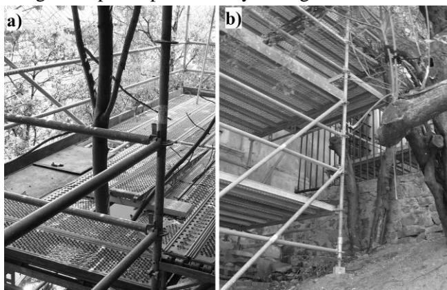
Fig. 4. The east elevation a) tree in the immediate vicinity of the facade b) the fence perpendicular from the facade
