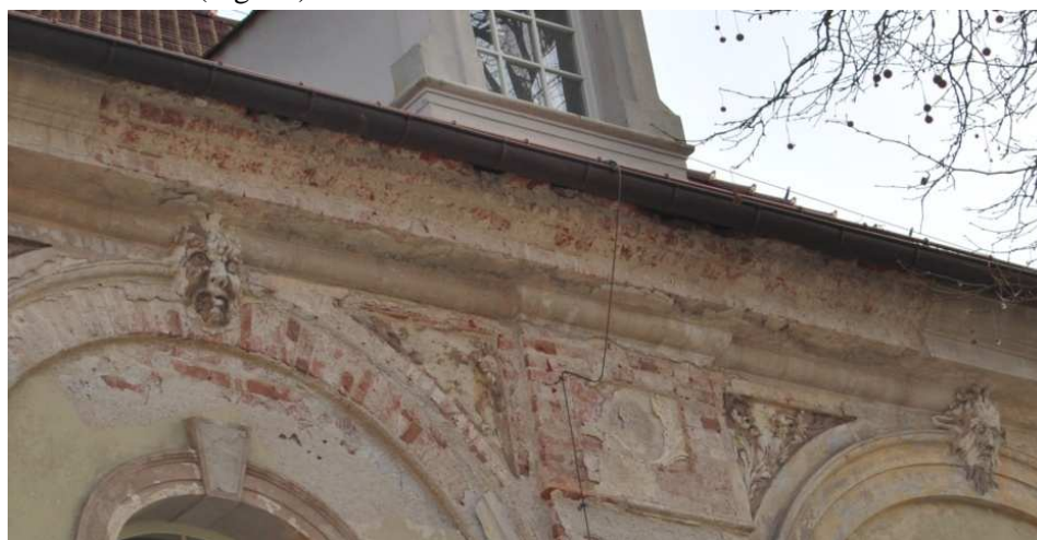
Fig. 10. Deteriorating east façade (fot. W. Sokołowski)
