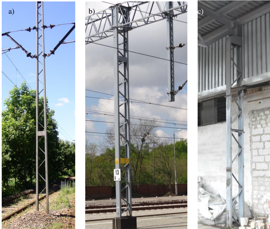
Fig. 1. Examples of investigation columns: a) tram railway support, b) intermediate column in railway traction gate, c) in industrial building
