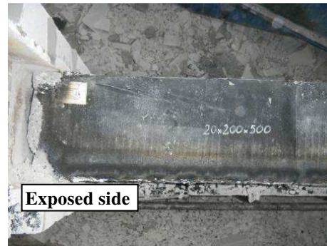
Linear joint seal No. IV extent of thermal degradation – 45 mm
