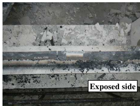
Linear joint seal No. I extent of thermal degradation – 16 mm
