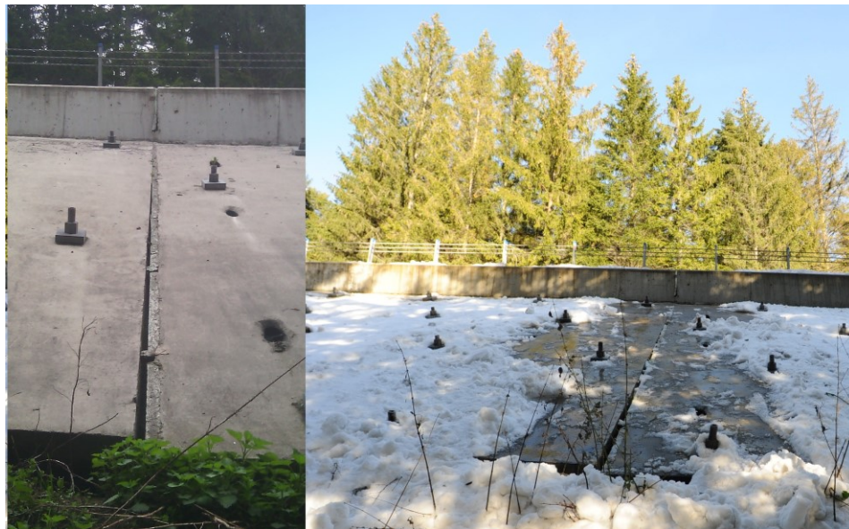
Fig. 3. Section of the failed slab of the anchored retaining structure
