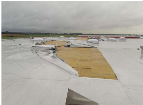
Fig. 5. Damage to the roof of the hall no. 2. A detached membrane in the perimeter zone, exposed thermal insulation
