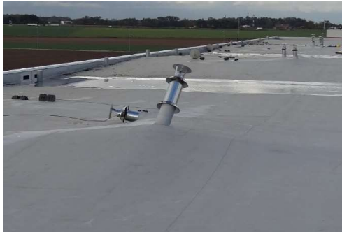
Fig. 4. Damage to the roof of the hall no. 1. Overturned roof ventilation chimneys
