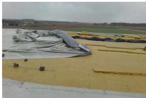
Fig. 3. Damage to the roof of the hall no. 1. A detached membrane in the perimeter zone, exposed thermal insulation
