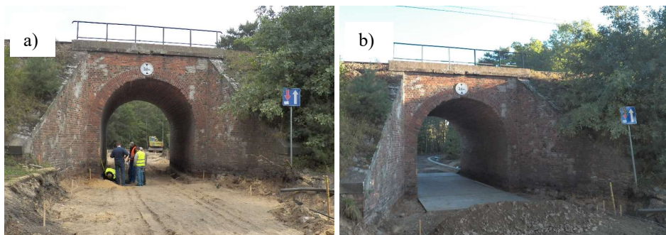
Fig. 4. View of carrying out works on the bridge structure: a) preparing the road bed, b) preparing the expansion slab under the viaduct
