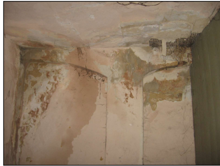
Fig. 8. Part of the eastern wall on the upper floor. Very damp wall and ceiling. Visible mould
