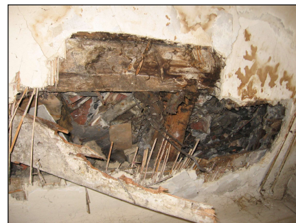
Fig. 11. Section of the ceiling above the ground floor. Moisture of ceiling beams, defects in the ceiling fillings
