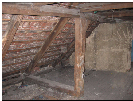
Fig. 12. Numerous defects in the construction of the truss. Purlins and rafters strongly bent
