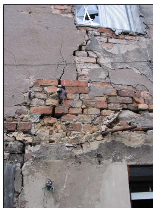
Fig. 7. Part of the southern elevation. Loose brickwork, defects in the joint
