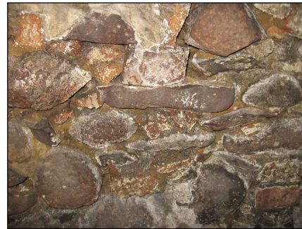
Fig. 5. Part of the stone wall of the basement. Wall salting and moisture
