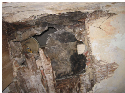
Fig. 10. Section of the ceiling above the ground floor. Missing part of the ceiling, other beams corroded
