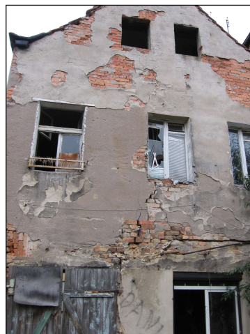
Fig. 3. South elevation. Numerous cracks and defects in the wall structure
