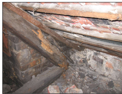
Fig. 13. Wet knee wall. The rafter ends are corroded, no wall plates, bent battens
