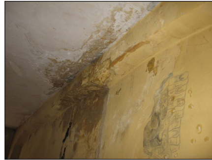
Fig. 9. Part of the eastern wall on the upper floor. Strong moisture of the wall and ceiling due to leakage of the valley
