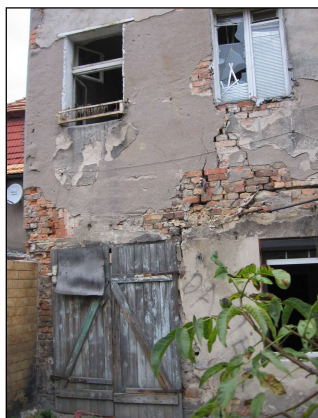
Fig. 6. Part of the southern elevation. Crack near the south-west corner
