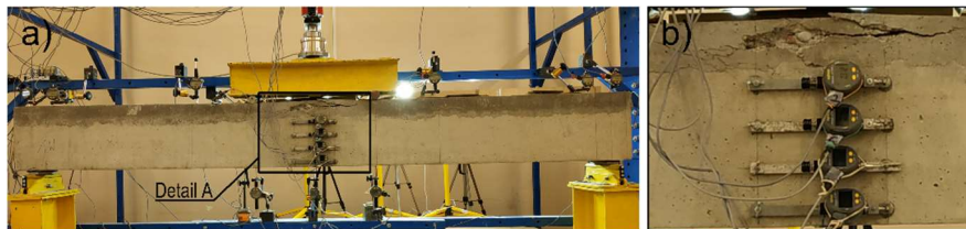
Fig. 6. View of test item after test (own photo), a) general view, b) detail – A
