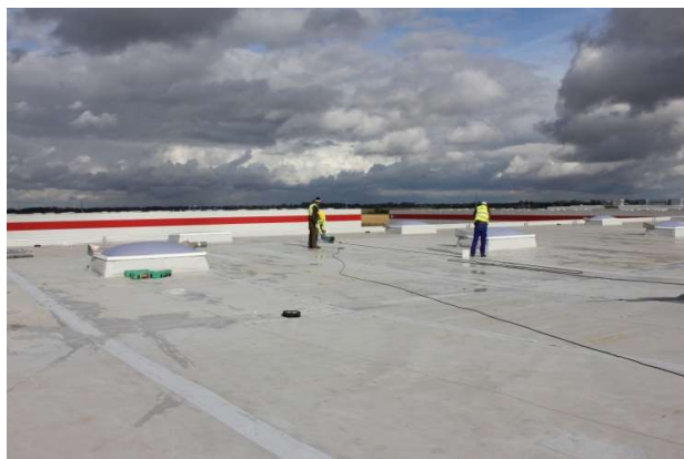
Fig. 2. Ponding water due to incorrect roof falls [Photo by Barbara Ksit]
