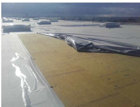
Fig. 1. Damage to roof sheathing caused by the action of wind [13]
