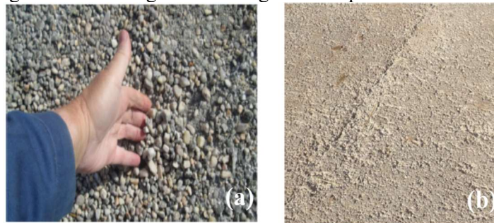
Fig. 6. Raveling due to (a) poor paste -aggregate bonding (b) insufficient compaction [12]
