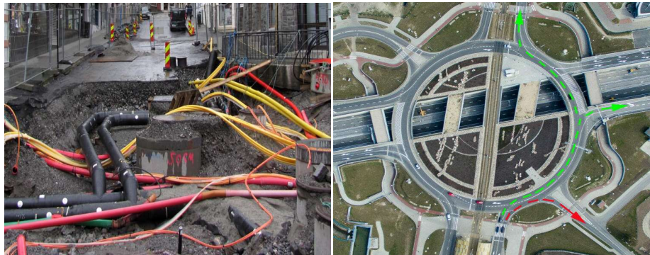
Fig. 13. Location of cables and pipes of underground integrated installations introduced into existing development [26]
