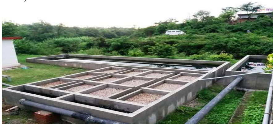
Fig.7. Commercial wastewater constructed wetland wastewater treatment system
