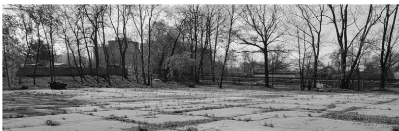
Fig.3. Inner central part of the study area before pavement demolition in 2020. Fot. PWIK archive
